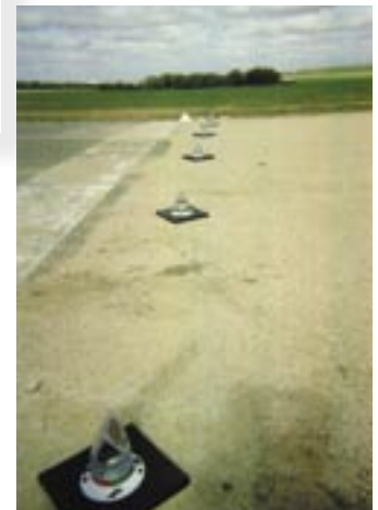
Solar powered temporary airstrip lighting, Loxton Council Airport, South Australia.
